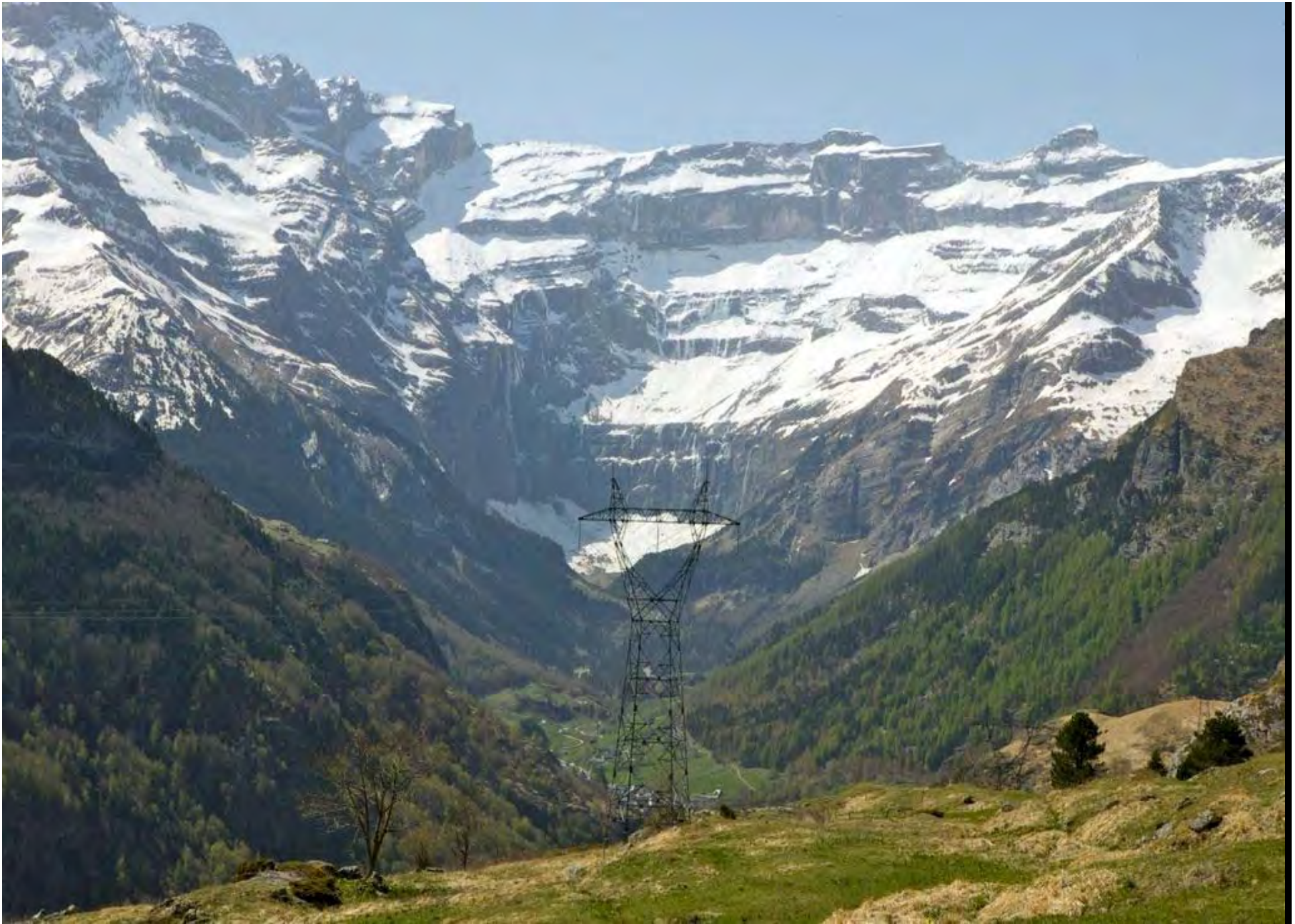
Electrical tower on the pastoral plateau of Saugué; on the background the circus of Gavarnie
